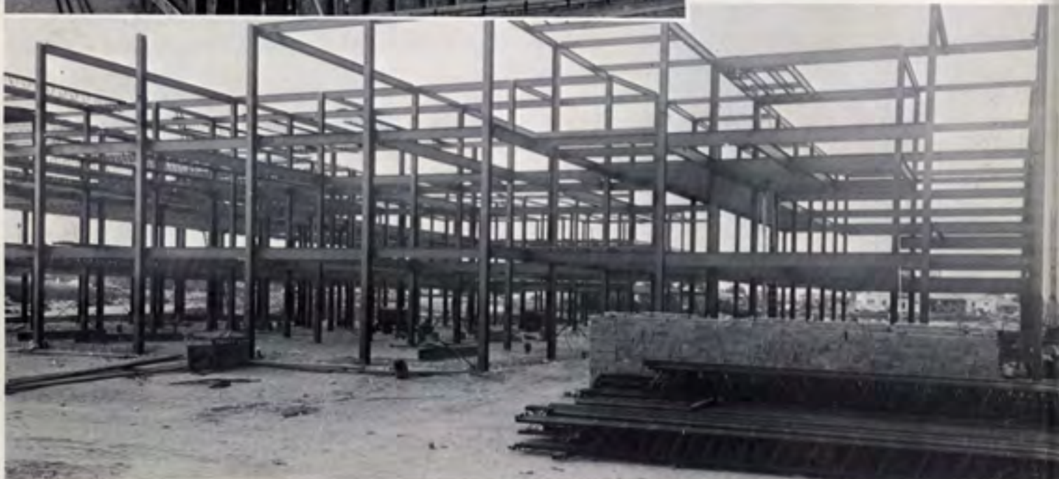
October 27, 1961 — Steel girders rise skyward to form a framework for the future — a new dimension.
